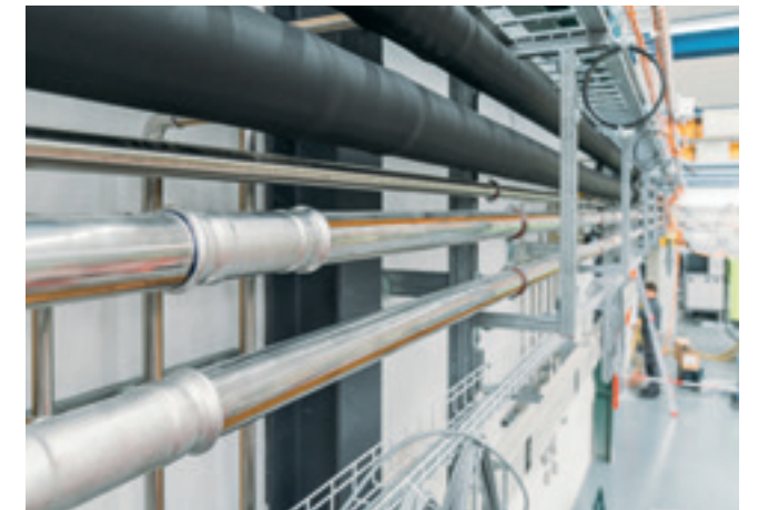
↑ Economical and corrosion-resistant system for cooling lines.
